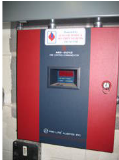
Fire Alarm System Control Panel
