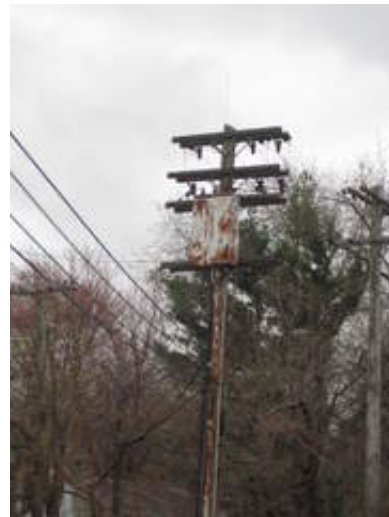
Pole Mounted Transformer
