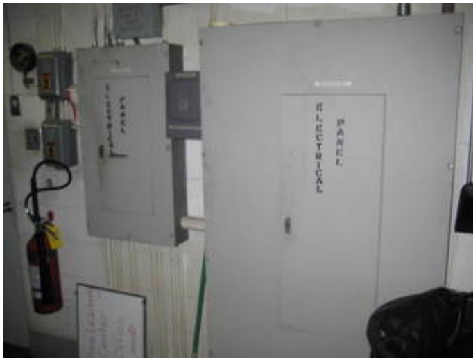
Main Electrical Distribution Panel
