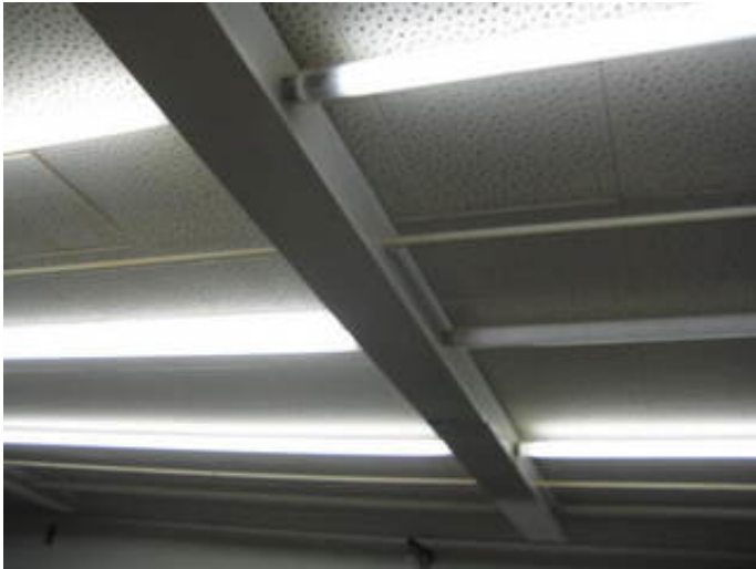
Typical Classroom Fluorescent Light Fixtures
