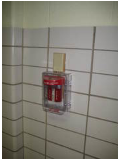
Fire Alarm Manual Pull Station
