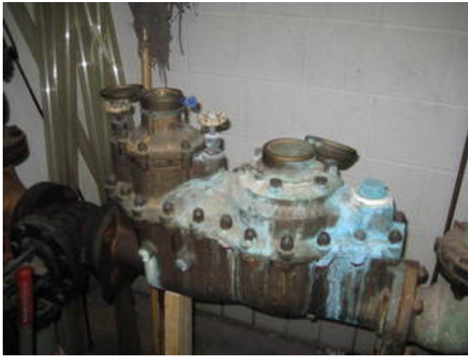
Incoming Domestic Water Service Meter
