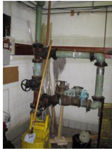
Incoming Domestic Water Service Line
