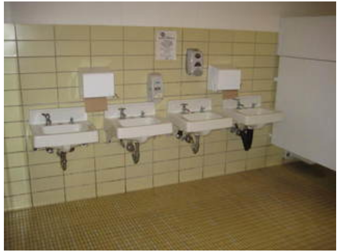
Non-ADA Wall Mounted Lavatories
