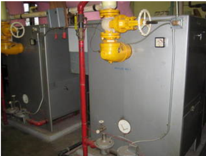
Natural Gas Fired Heated Water Boilers
