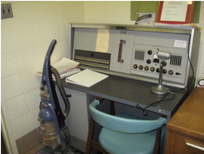
Outdated Building PA System
