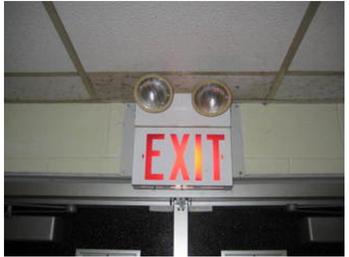
Illuminated Exit Sign and Emergency Egress Light Fixture
