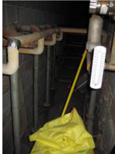
Sanitary Waste Piping
