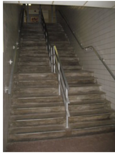
Non-Compliant Stair to Lower Level Classrooms
