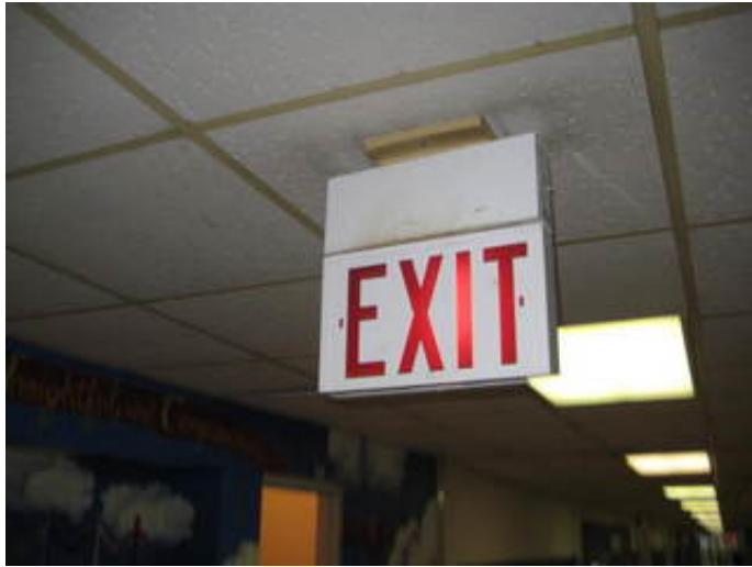
Illuminated Exit Sign
