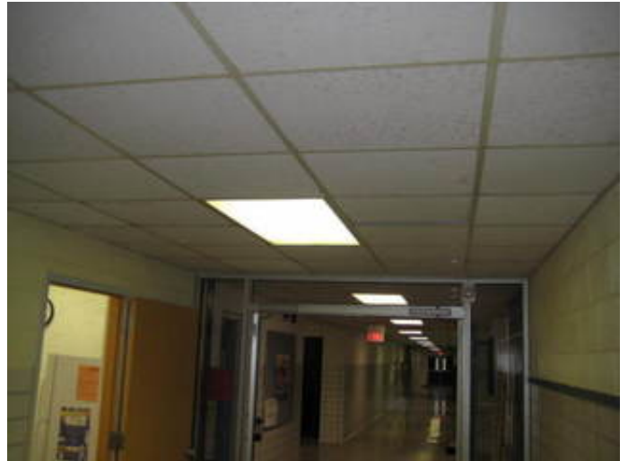
Typical Corridor Fluorescent Light Fixtures
