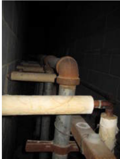
Sanitary Waste Piping
