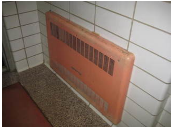
Heating Water Cabinet Heater
